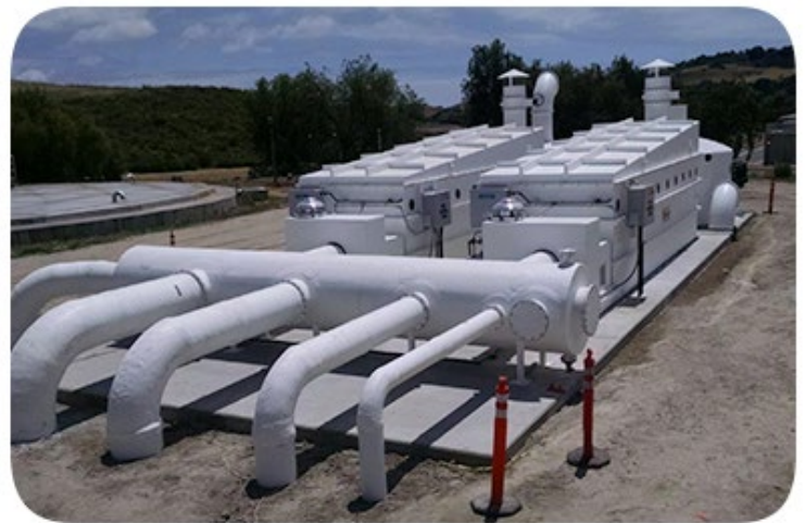
I-BOx® 8025, SMWD's 9.0 MGD Chiquita Water Reclamation Plant
